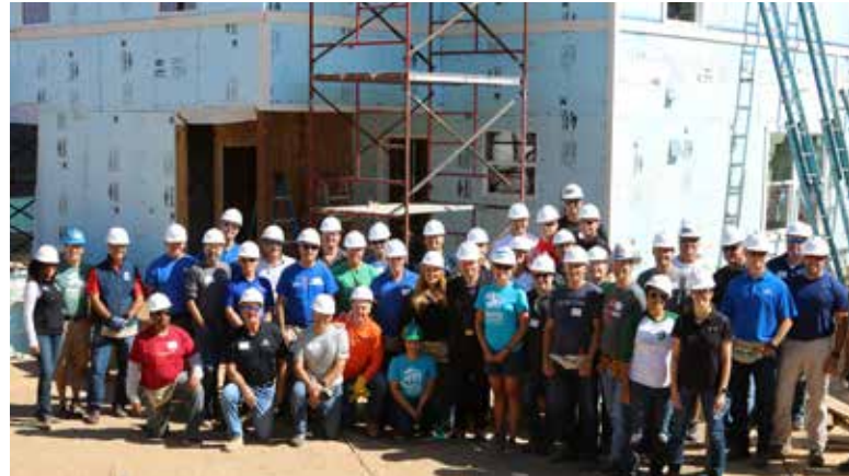
Above: President and CEO Joe Ellis co-hosts the sixth annual CEO build with Habitat for Humanity of Metro Denver's Executive Director and CEO Heather Lafferty. The event encourages Denver-area CEOs to exchange their suits and ties for hard hats and hammers.
