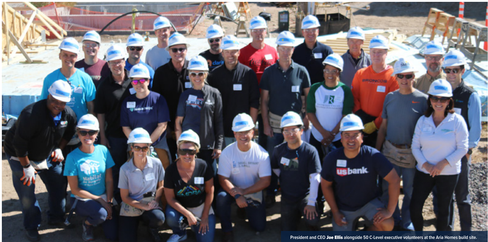
President and CEO Joe Ellis alongside 50 C-Level executive volunteers at the Aria Homes build site.
